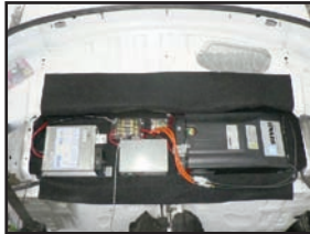
Components in place of fuel tank
